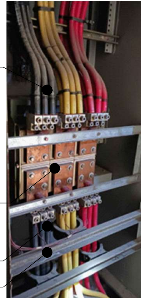
MAIN AIR CIRCUIT BREAKER (REAR VIEW)
