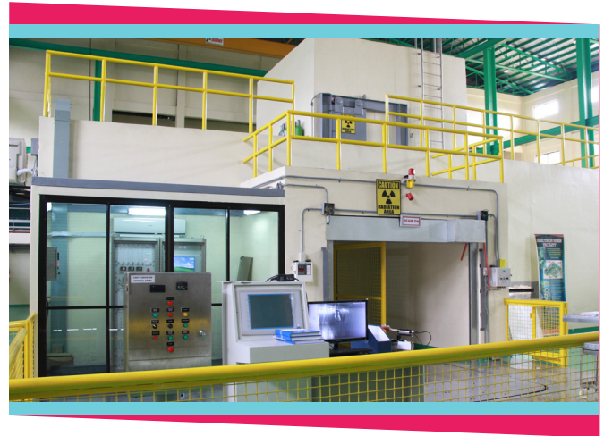
Electron Beam Irradiation Facility
