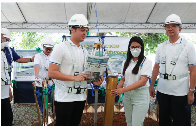
DOST Secretary Fortunato T. de la Peña (rightmost) with ISI President Paul Francis Juat (leftmost) at the official groundbreaking of the Tanay Electron Beam and Cold Storage Facility in Brgy. Sampaloc, Tanay, Rizal
