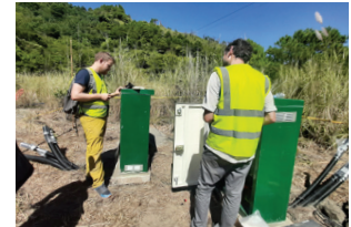
Installation of PRIME cabinets which contains the main circuit boards and control systems
