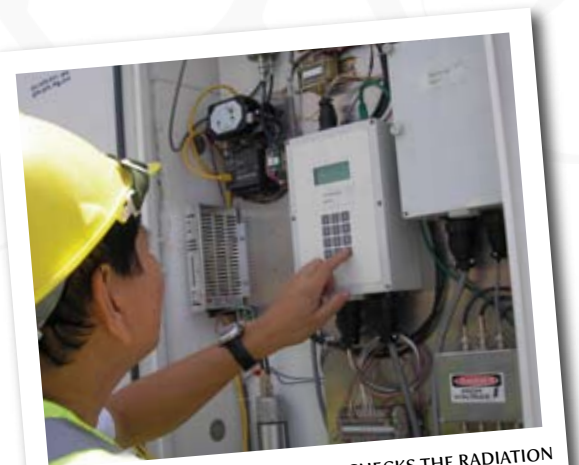
PNRI ENGINEERING SERVICES STAFF CHECKS THE RADIATION PORTAL MONITOR INSTALLED AT PORT AREA, MANILA
