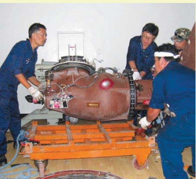
Decommissioning activity in Davao Doctors Oncology Center teletherapy machine
