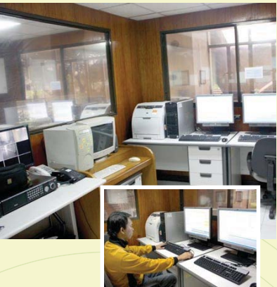
Mirror Central Alarm System at PNRI
