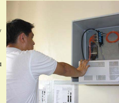
Preventive maintenance of the ICT component of the radiation portal monitoring system
