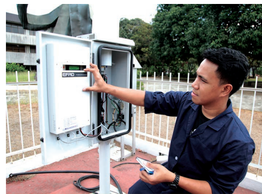
Maintenance check-up of the EFRD-3300 real-time online radiation monitoring system
