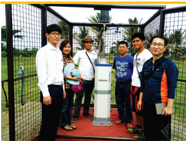
The EFRD3500 real-time environmental radiation monitoring station installed by the project staff of SI Detection Co., South Korea and PNRI at the PAGASA Aparri Station in Cagayan
