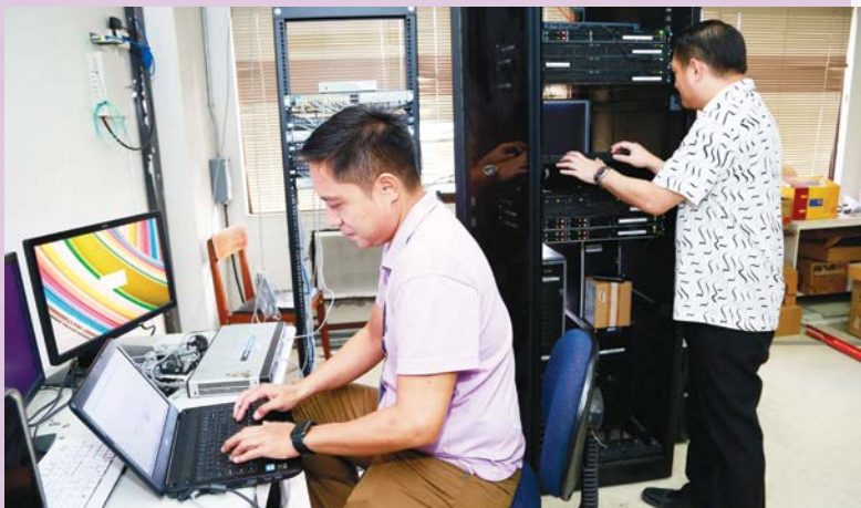
IT staff of the Management Information System Section at the PNRI server room
